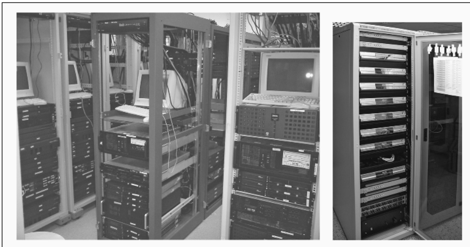
Figure 3-1 Cabinets and racks in a data center.
